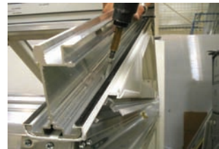
When a gable frame is used, the end rafter top and bottom bolts become redundant. Screw fix the end rafter to the head of the gable window as shown at 300mm centres.
